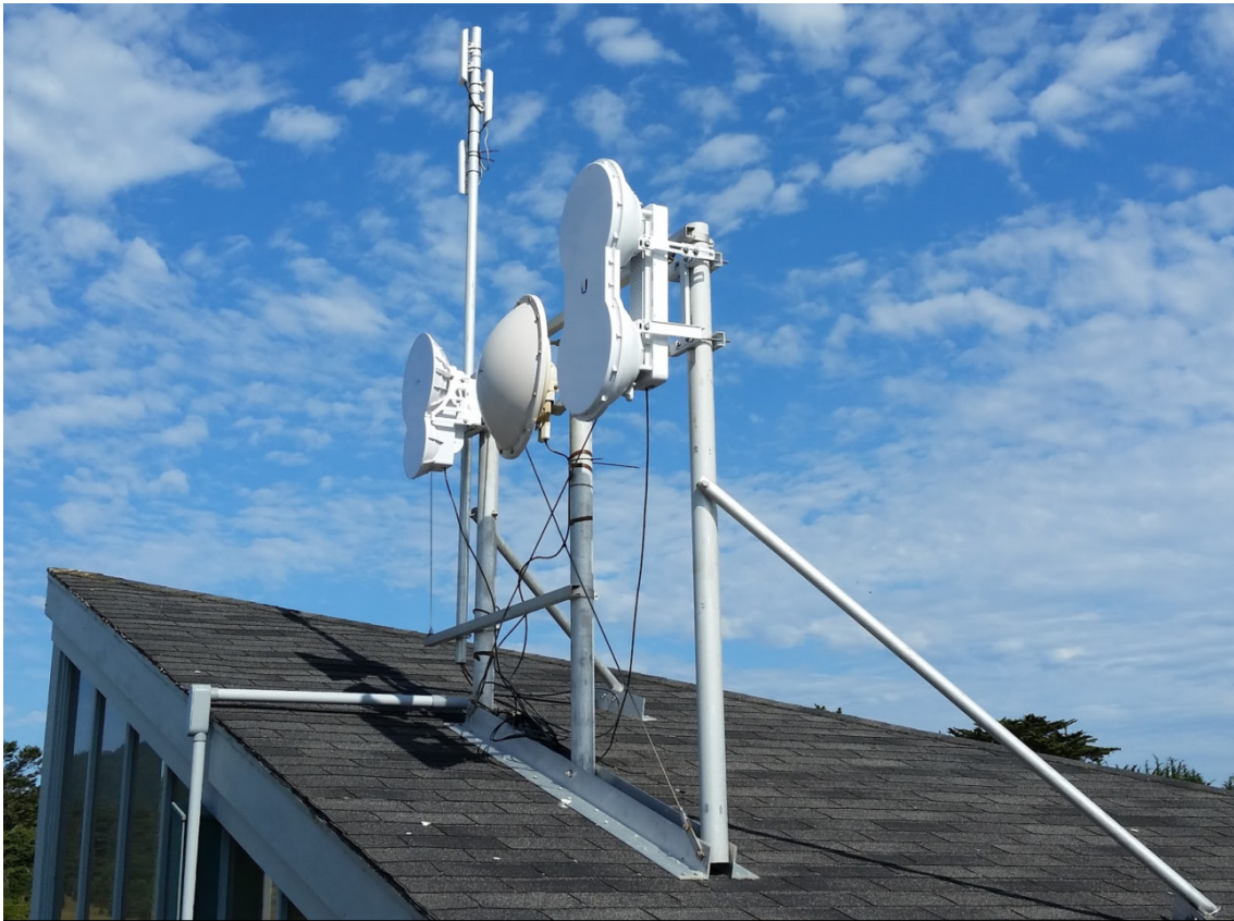
Figure 2.11: MES site — the roof of our 2nd fiber-fed site.
