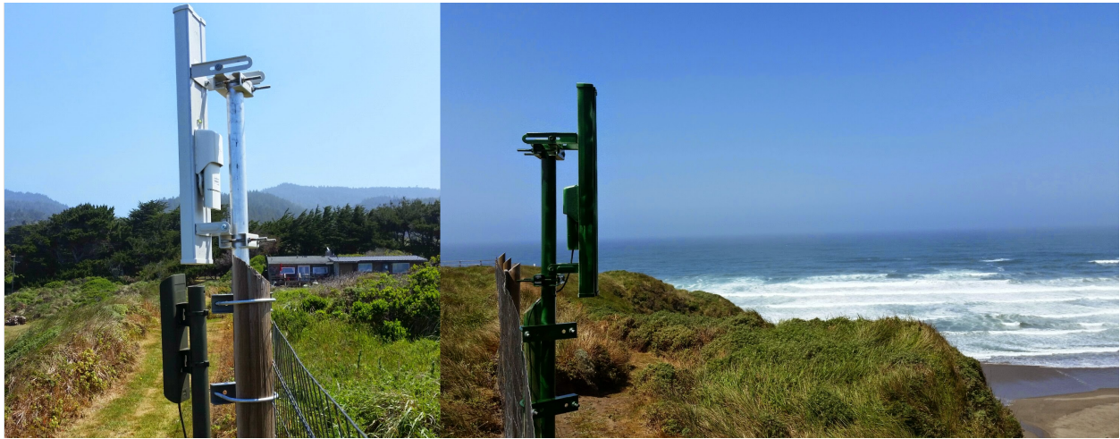
Figure 1.5: Small distributed relay site with low visual impact.
