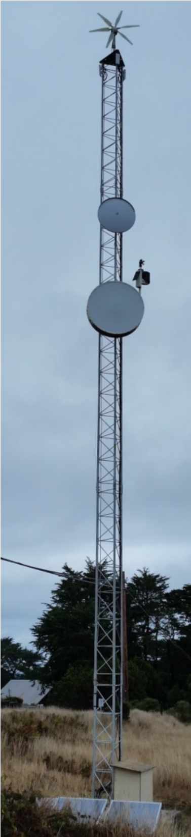
Figure 2.18: Navarro site — FurtherReach’s tower powered by a hybrid of renewable energy sources.
