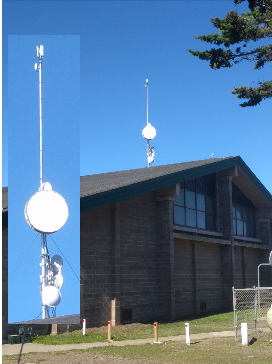
Figure 2.13: FurtherReach’s relay on the roof of the Point Arena high-school’s gym.
